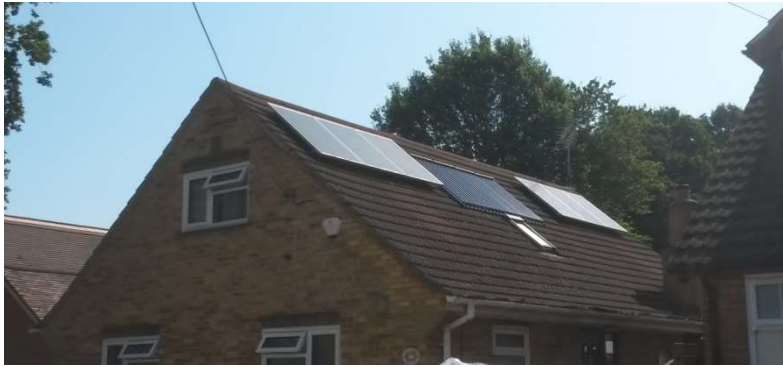
Roof mounted solar electric panels (outer panels) and solar water heating panels (middle panels)
